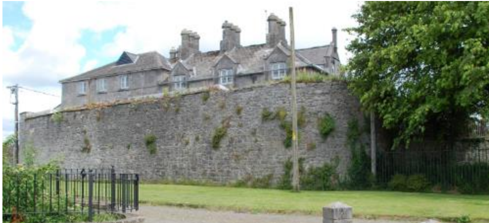
Plate 14-41. Possible nineteenth century boundary wall adjoining medieval tower at north-western end of Villiers Almshouse, protected structure (RPS 001)
