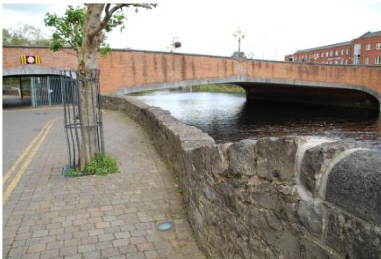
Plate 14-63. Wall at north between Baal's Bridge and Abbey Bridge, which will be rebuilt as part of the flood defences
