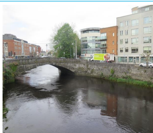
Plate 14-27. View of Baal's Bridge, facing west from Lock Quay with Area 10 to right
